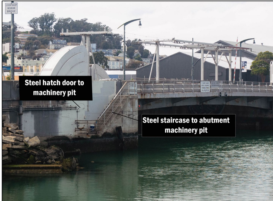
Figure 4.B-3 Character-Defining Steel Staircase Leading to Abutment Machinery Pit and Sidewalls of Concrete Abutments, at Southeastern Corner Leading to Steel Hatch Door, Facing Northwest
